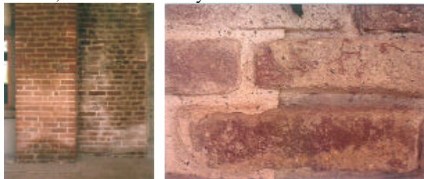
Figure 8: CCR: a) rising damp; b) damage of the repointing
