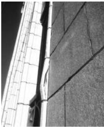
Figure 2: Buckling of terra cotta
