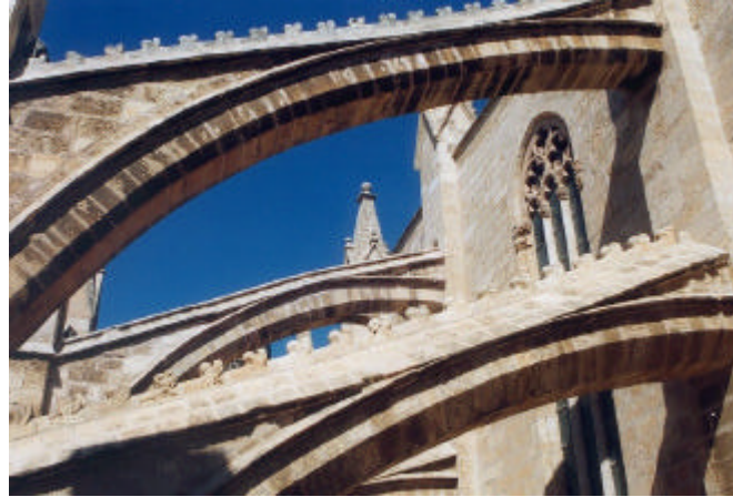
Fig 2.- Apparent deformation of flying arches
