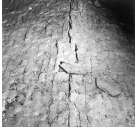
Fig. 4: Extradossal cracks at the key section [12]
