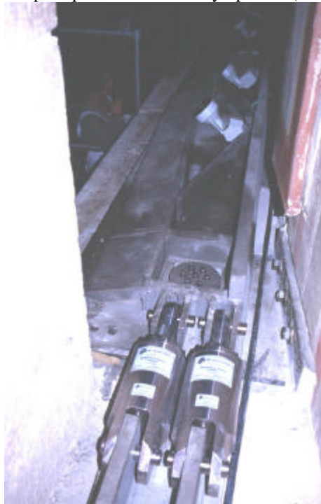
Fig. 3 : The installed STUs.
