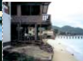
(top) This newly constructed building at Carriacou is on the beach and is very vulnerable to hurricane waves, 2000
