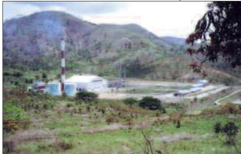
Kanudi Diesel Power Station
