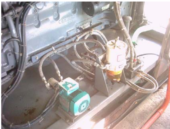
Figure 2: Fiji Rural Electricity Generation adaptations: special pump and filter.
