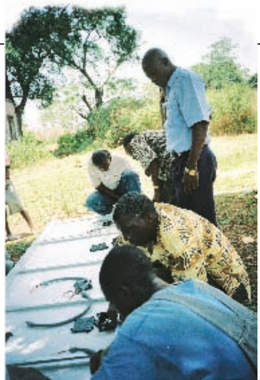
Electrical cabling of solar panels and the installation of solar systems by participants as part of practical field-work organized by UNESCO in Bamako (Mali) in 2003
